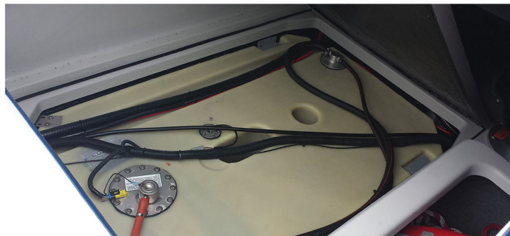
Figure 2. A ballast bag is pliable and collapsible, and often has two connected hoses in order to fill and drain the ballast (left). It was observed that the hoses could lift the drain connection above the lowest part of the ballast bag, resulting in a significant amount of residual water in the ballast bag (right). A hard ballast tank (bottom) fills an entire compartment, even when not full, and is generally inaccessible without tools. Photo credit: Tim Campbell.
